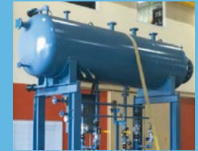
Newly installed condensate recovery tank at our Manati Site
