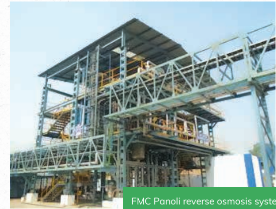
FMC Panoli reverse osmosis system
